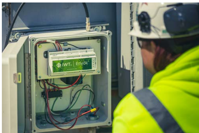
Figure 2. A wireless node installed at an operation's pump-back station allows for remote monitoring.
